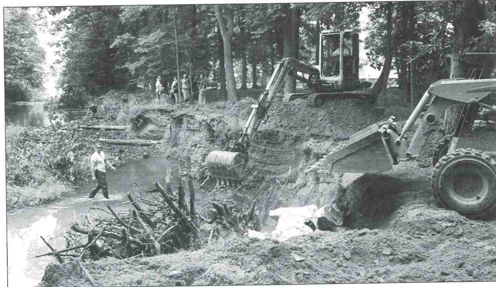
Mill Creek’s six-foot-high, almost-vertical banks of soft loamy soil meant this site was extremely vulnerable to erosion, with the loose soil polluting the stream and degrading water quality from this point on. Improvement work included re-grading the streambanks (shown in process here) to reduce the severity of their slope.
