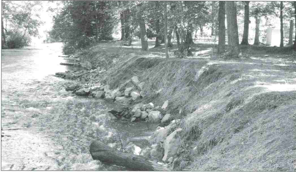
The nearly completed project features re-graded streambanks; logs, stone, and tree roots added to slow the force of the water; and new grass planted to stabilize the bank.
