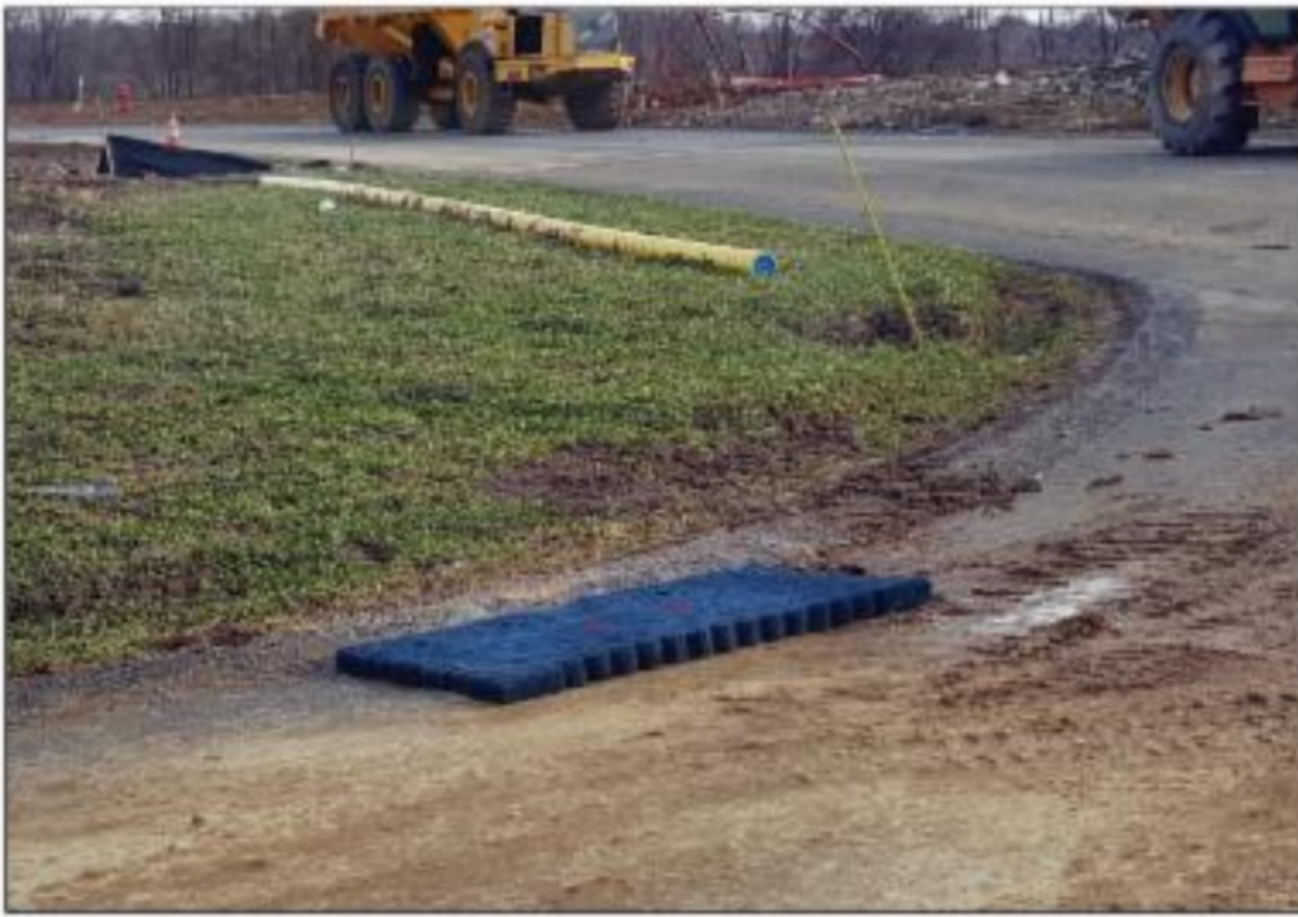
Newly installed BlackHawk Inlet Filter Mat
