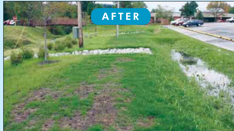
The asphalt in the "before" photo has been removed and replaced with a grassed buffer and swale. These will help absorb stormwater runoff coming from the rest of the parking lot before it reaches the creek.
