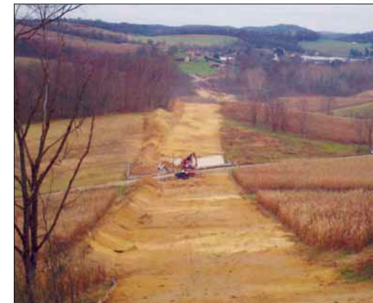
The Appalachian Gateway gas line construction site is winterized by covering disturbed earth with straw mulch.
