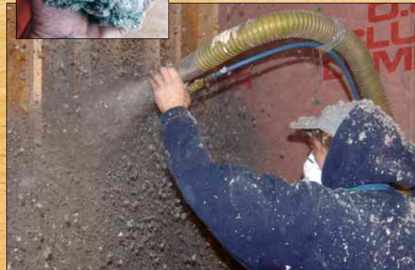
The recycled newspaper insulation is applied to the inside walls prior to paneling.
