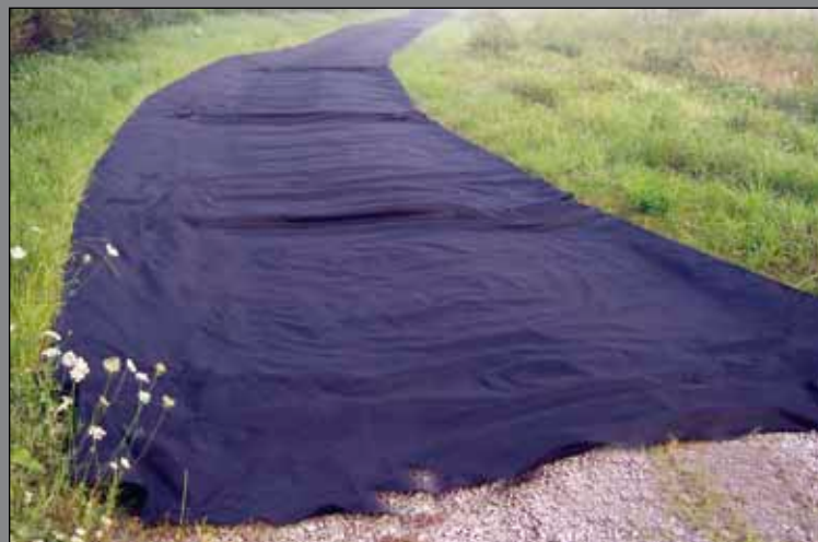
Due to its lower elevation, Thomas Road was covered with geotextile to help keep mud from coming up through the fill.
