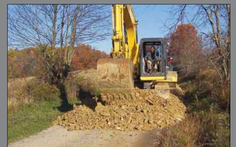
Bridges Road required three feet of fill to bring it up to a level which would disperse stormwater effectively.
