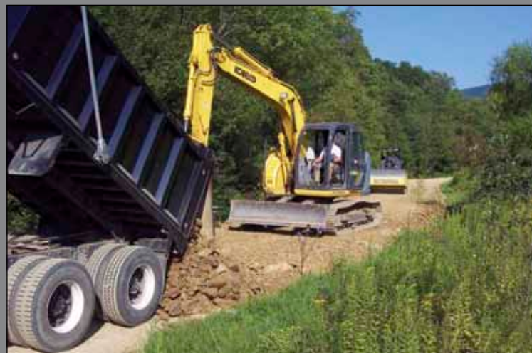
Fill is applied over the geotextile layer on Thomas Road to make the road's level higher than the neighboring creek.
