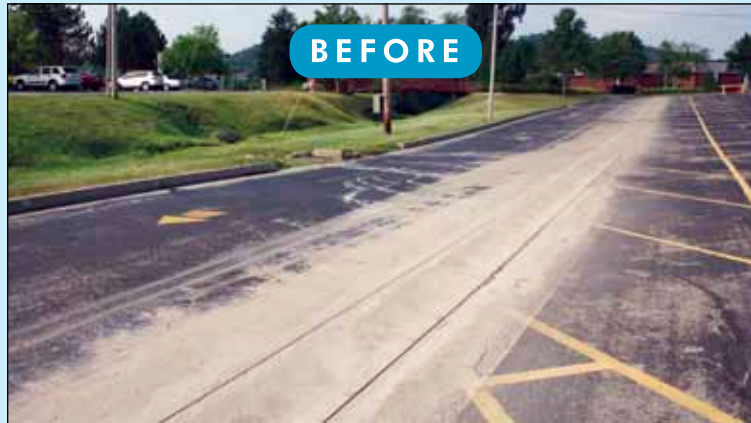
Acres of asphalt near the creek allows for great volumes of stormwater runoff to pour into the creek at a high speed.
