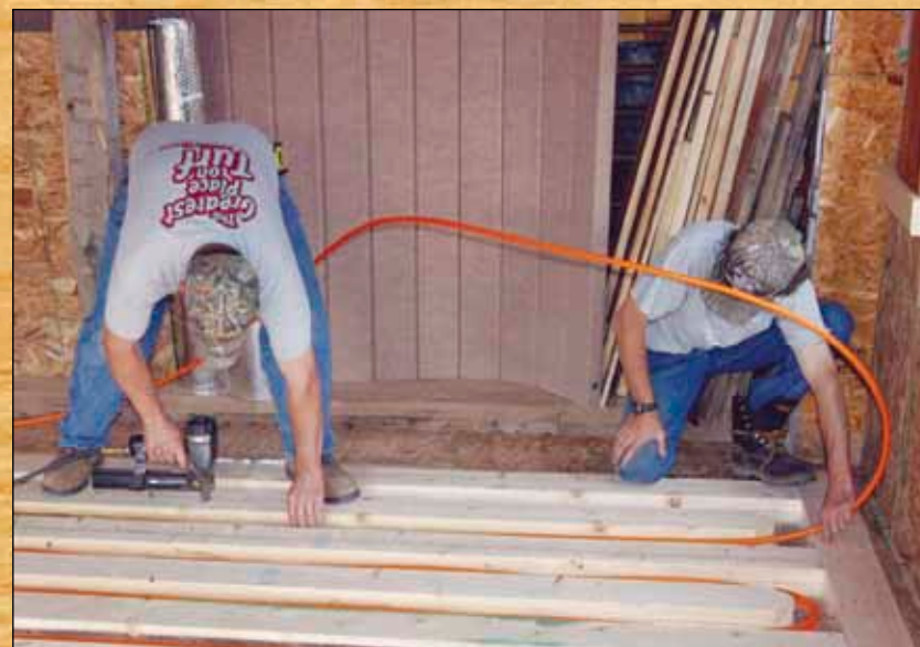
Extending the geothermal heating and cooling system to work in the newly enclosed deck addition.
