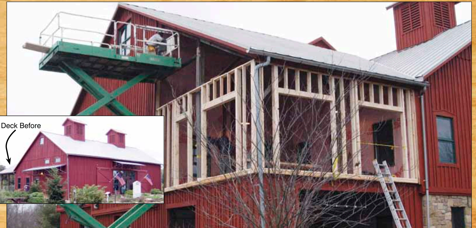
Framing in the last remaining barn deck to add more interior meeting space. The siding style and color will match the rest of the barn.
