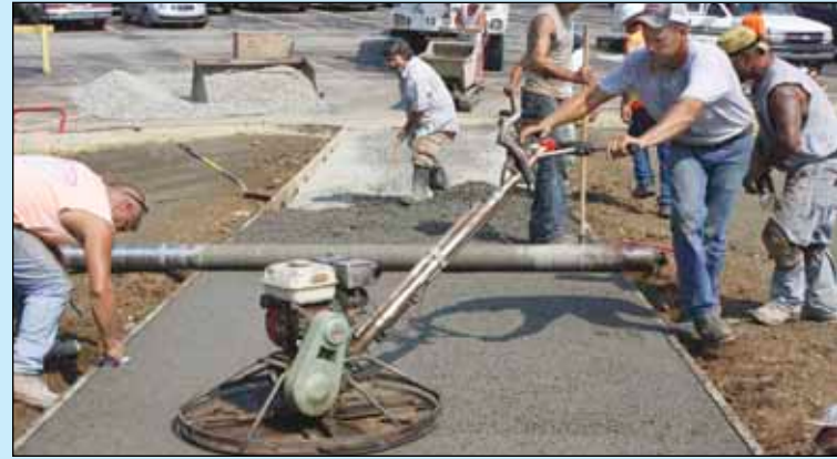
Workers install a porous concrete sidewalk near the creek. When finished stormwater will be able to pass through the concrete into the ground.
