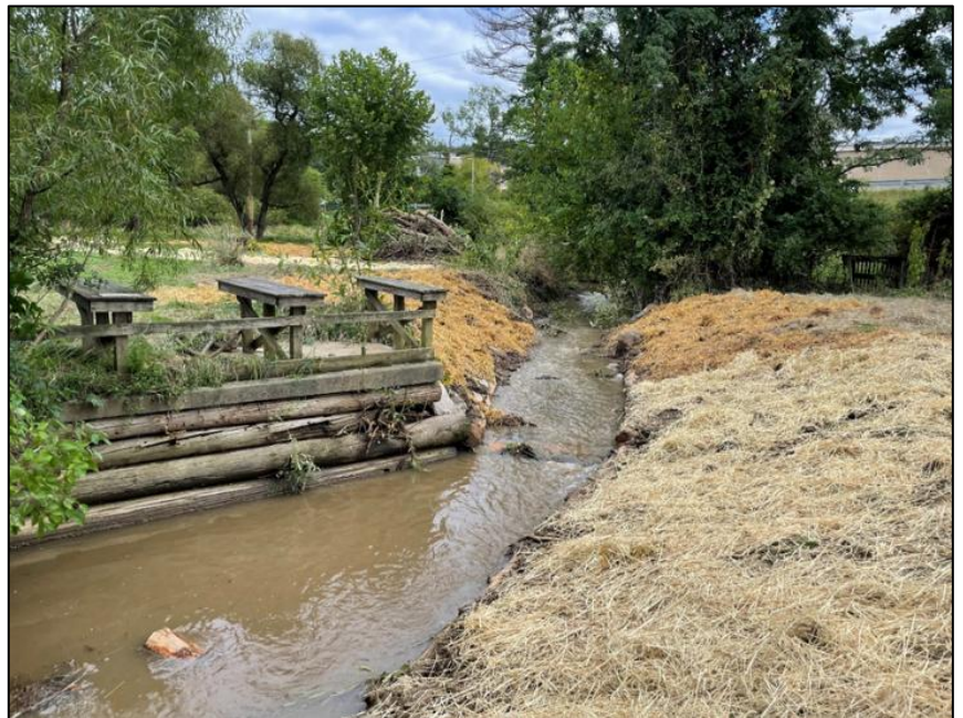
Site after debris was removed and structure was repaired and retrofitted. Banks were also graded and stabilized.
