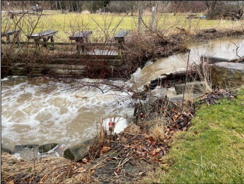
Site of collapsed bridge on top of in-stream structure. Debris is blocking stream flow and creating severe erosion along streambanks.
