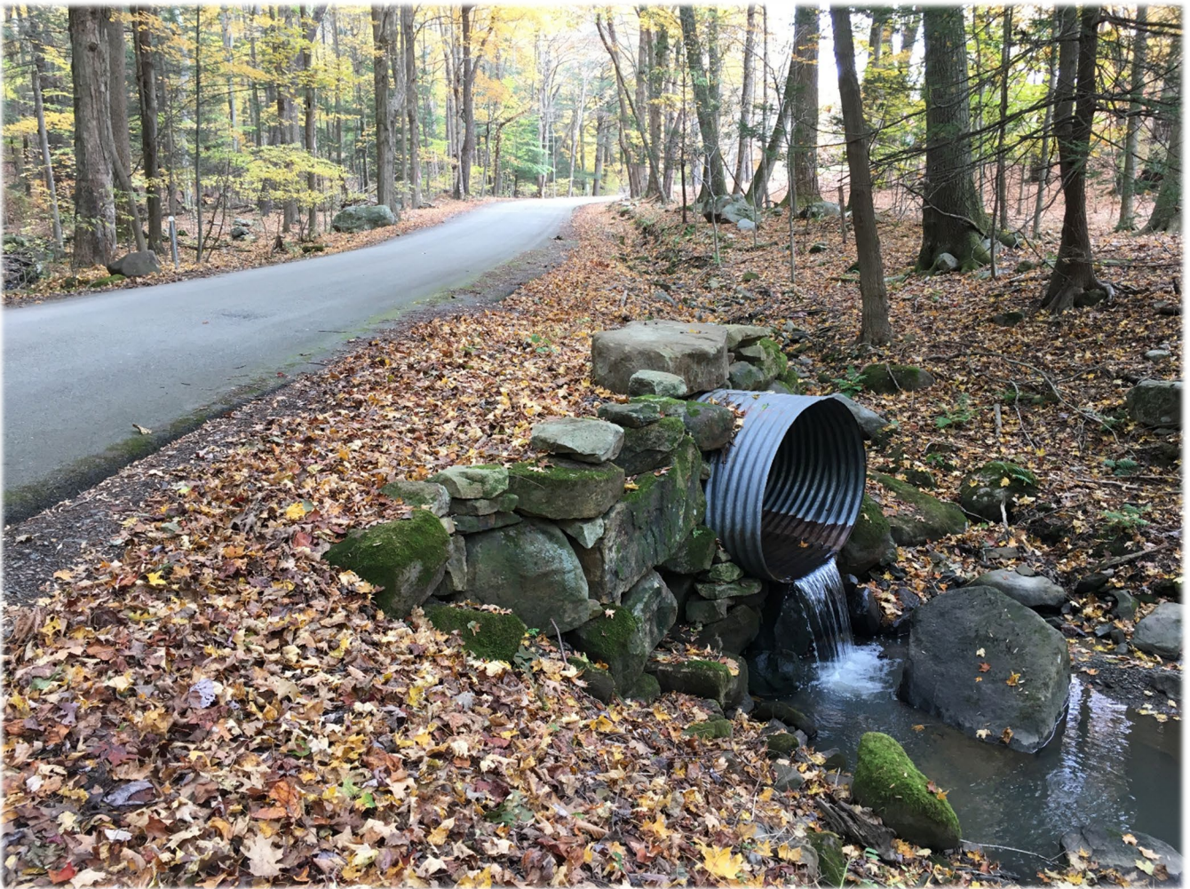
(Before): waterfall at the outlet of pipe impeding aquatic organism passage.
