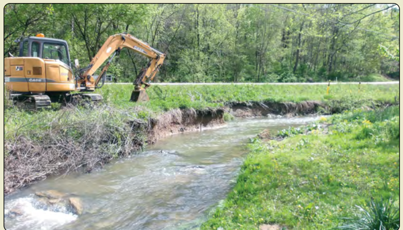
Before: Streambank erosion threatening SR 366 (Greensburg Road).
