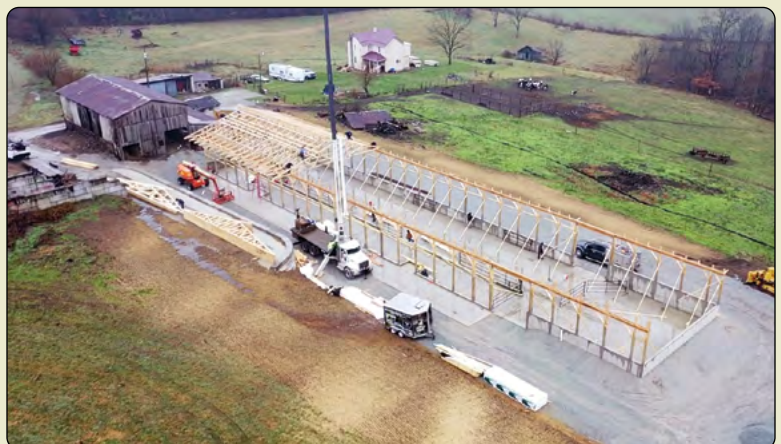
Ongoing construction of the 8,320 sq. ft. roofed animal heavy use area – installation of roof trusses, concrete work, and access road completed.
