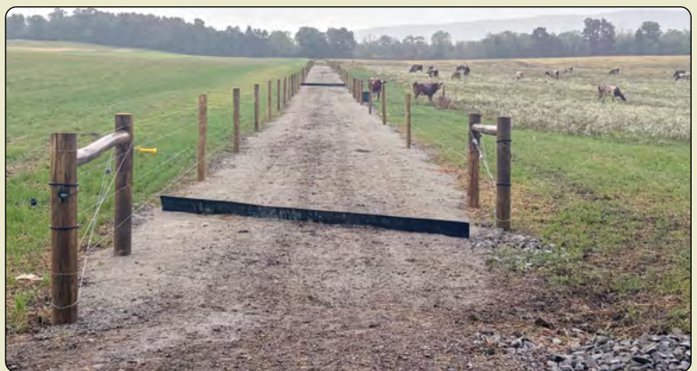
After: Stabilized animal walkway with conveyor belt diversions to prevent erosion of the surface, which will prevent sediment from entering Sewickley Creek.
