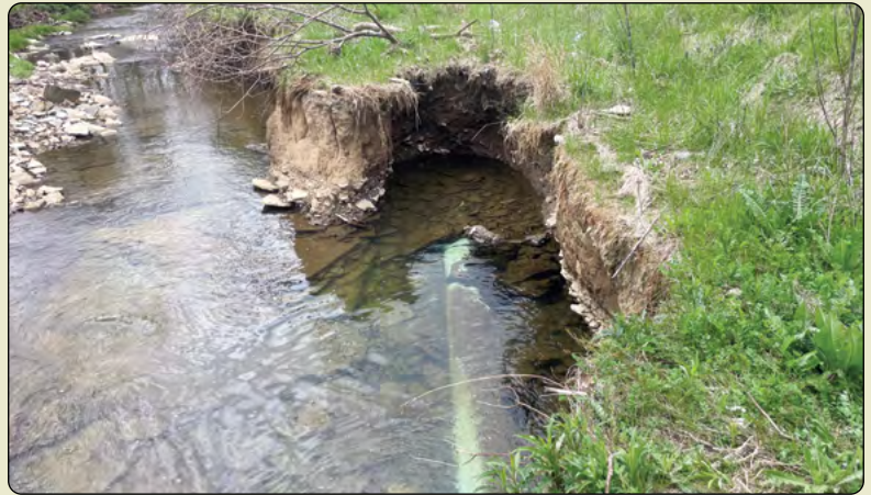
Before: Severe streambank erosion around exposed sanitary sewer line.
