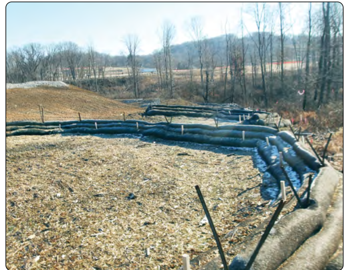
A compost filter sock sediment trap acting as a perimeter control containing loose dirt at the Mamont 138kV Power Line disturbed area.
