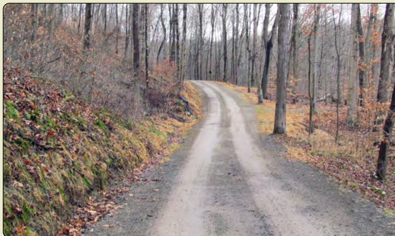
Before: Narrow roadway with little to no drainage.
