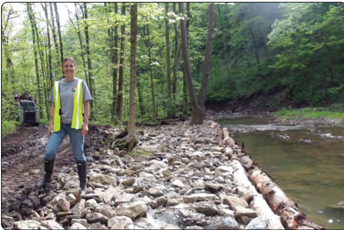
District Watershed Specialist Kylie Schultz inspected the Cedar Creek streambank stabilization project during construction.
