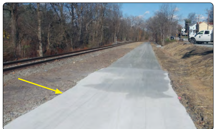
For safety, this section of the Five Star Trail was relocated farther away from the railroad tracks.
