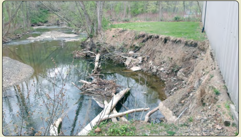
Before: Severe streambank erosion threatening the back of the Style-Rite Kitchens building.
