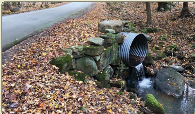
Before: Pipe outlet waterfall impeding aquatic organism passage.
