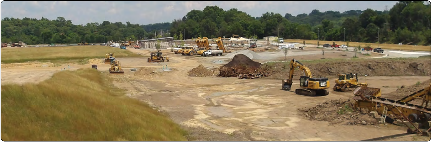
Construction progress overview of the Hempfield Township Municipal Complex and Weatherwood Park.
