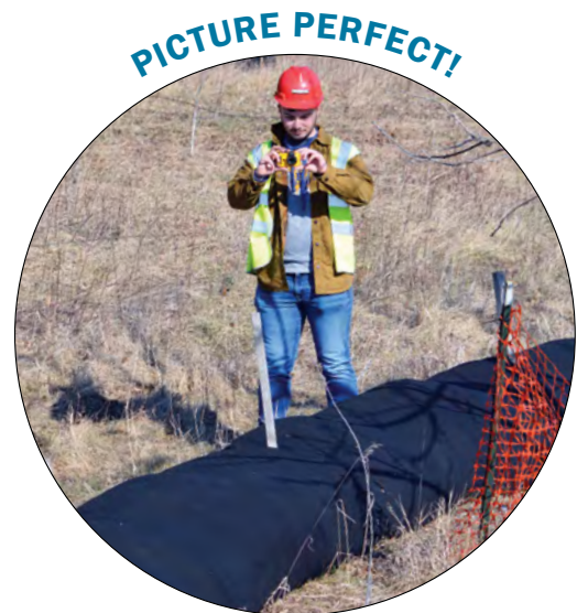
Jared Meharey photographs a sediment control filter sock during the construction of Weatherwood Park in Hempfield Township. This sock helps protect a natural wetland area from erosion sediment caused by the earth moving activities.
