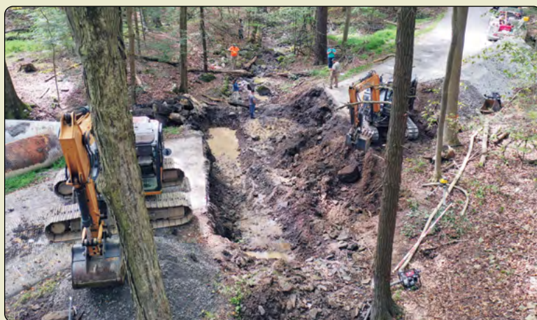
During Construction: A drone photo shows the roadway being excavated for the new structure.
